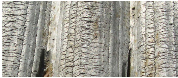
Figure 4: Fireside circumferential cracking of weld overlaid tubing
